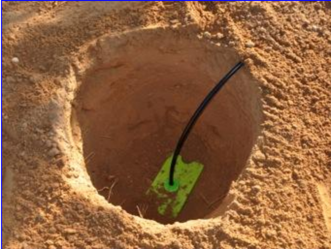
Buried diffuser in the pit with the 16mm connection tube
