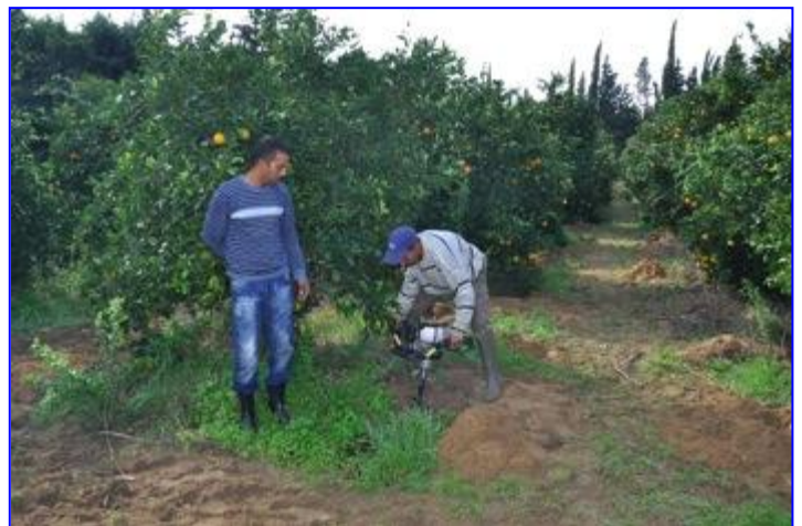
Installation of the buried diffusers for orange trees in Beni Khaled, Cap Bon North of Tunisia
