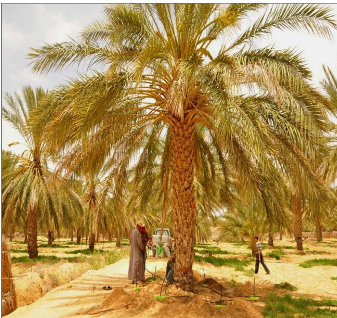
Installation of buried diffusers for dates palm trees in a private plantation in the oasis of Duos in the Desert (Kebili South of Tunisia)
