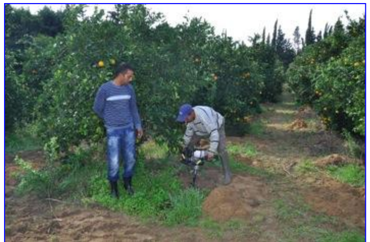
Installation of the buried diffusers for orange trees in Beni Khalled, Cap Bon North of Tunisia
