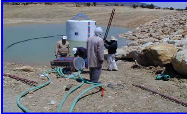
Connection of tubes to the floater and the tubes collector
